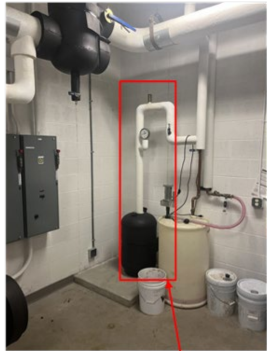
Existing Pressure tank, pressure gage and air vent.
